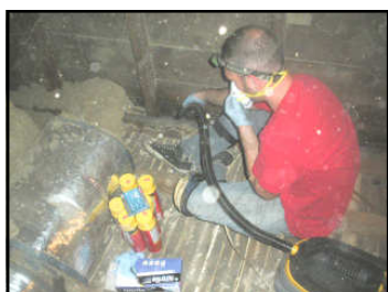
After clearing the attic, the air sealing team enters and begins spraying.
